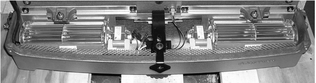
Photo 30 – Blower System (Ash Lip Cover Removed)
